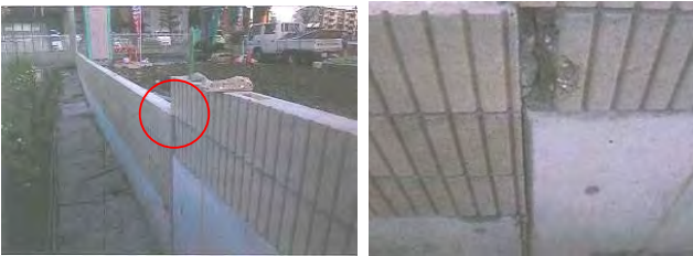
Fig.14 Deformation of retaining wall (case5)
