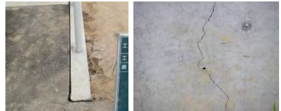
Fig.17 Deformation of retaining wall (case8)
