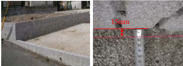
Fig.13 Deformation of retaining wall (case4)
