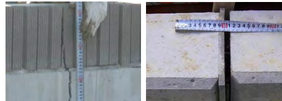
Fig.1 Deformations of retaining wall
