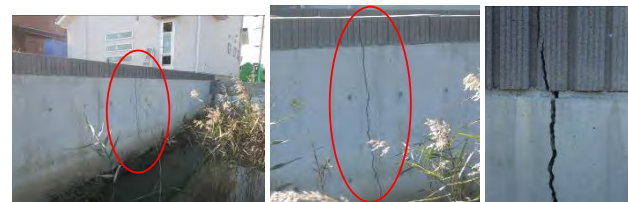
Fig.15 Deformation of retaining wall (case6)
