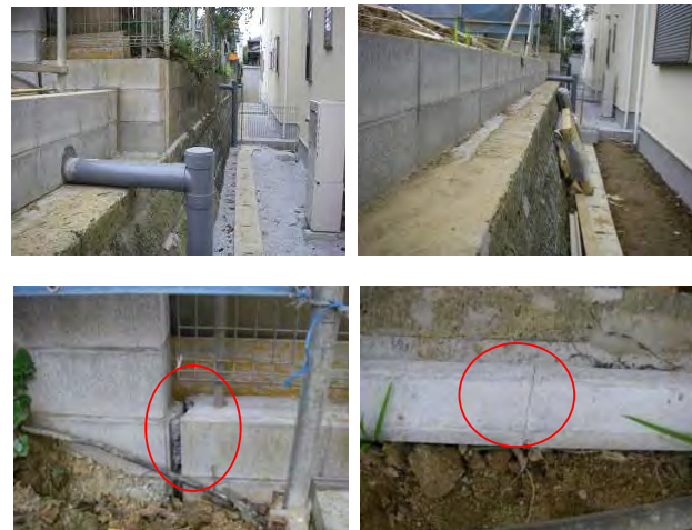
Fig.11 Deformation of retaining wall (case2)
