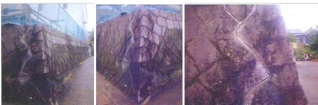
Fig.9 Deformation of retaining wall (case1)
