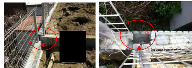
Fig.12 Deformation of retaining wall (case3)
