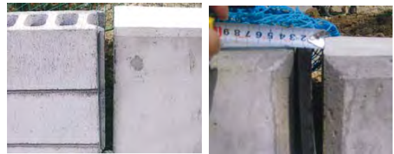
Fig.18 Deformation of retaining wall (case9)
