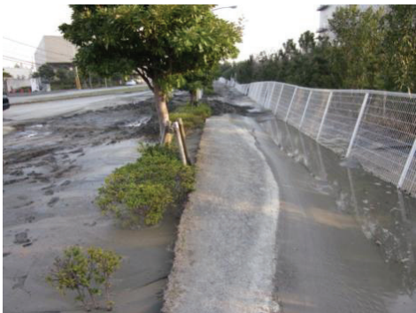
Photo.2 Ground surface covered by boiled sand (Chidori area)
