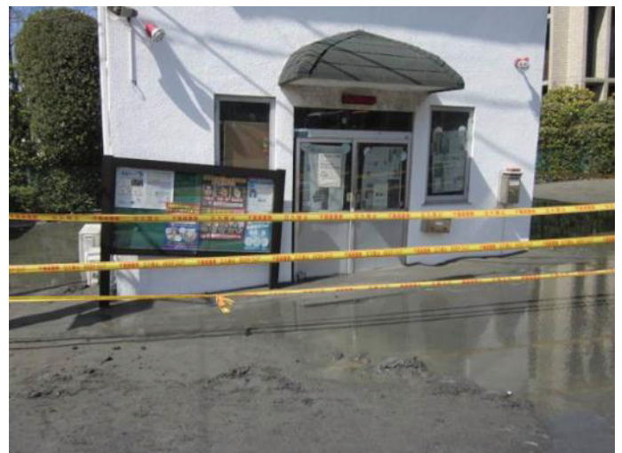
Photo.7 Uneven settlement observed at a police box
