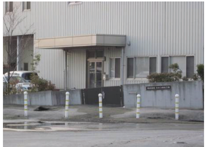
Photo.8 Inclined outer wall of a factory caused by sand boiling and subsidence
