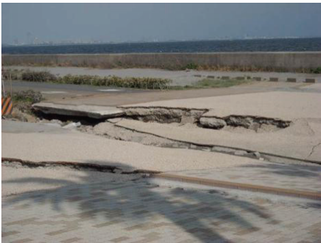
Photo.5 Sinking of soil near old levee (Hinode area)
