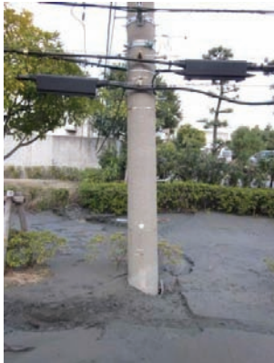
Photo.1 An electricity pole filled with boiled soil (Chidori area)
