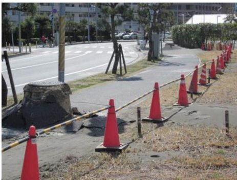
Photo.4 A protruding manhole in sidewalk (Hinode Area)
